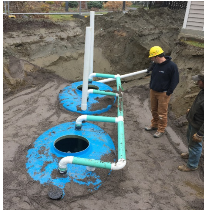
Grease Interceptor installed for pulper wastewater.
