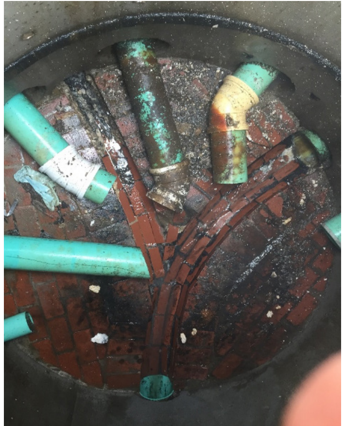
Which is causing the grease accumulation downstream? Sample them and find out!
