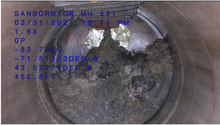
Clogged manhole in local sewer that caused a sewage backup in Sanbornton, NH.
