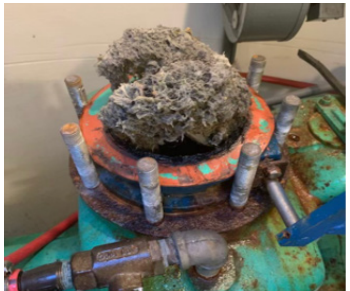
Clogged Check Valve in a WRBP Sewage Pumping Station located in Sanbornton, NH.
