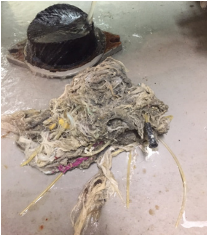
Wipe and catheter clog that was removed from a WRBP pump station in Laconia, NH.
