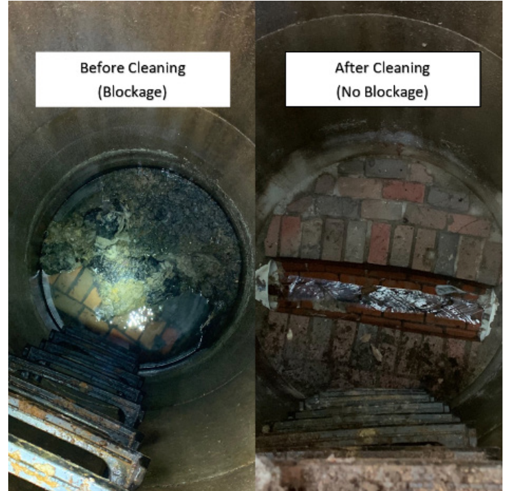
Before and after photos of clogged manhole in Sanbornton, NH. Wipes can already be seen accumulating in “After” photo.
